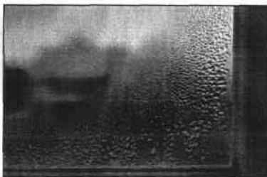
Condensation on the inside of a window-pane.
